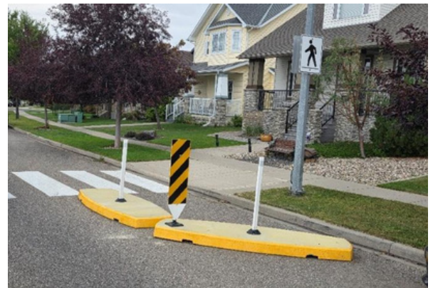
Figure 1 Example of an existing temporary traffic-calming curb installation at Riverstone Boulevard W & Riverview Crescent intersection in Lethbridge
